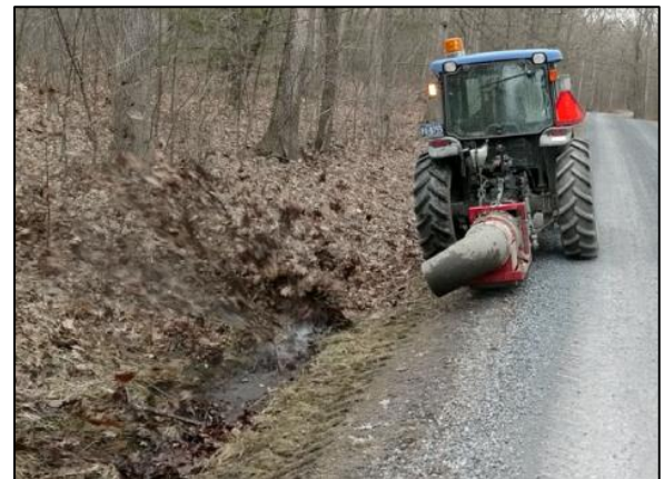
Leaf blowing is recommended to clean roadside ditches that are open and stable.
